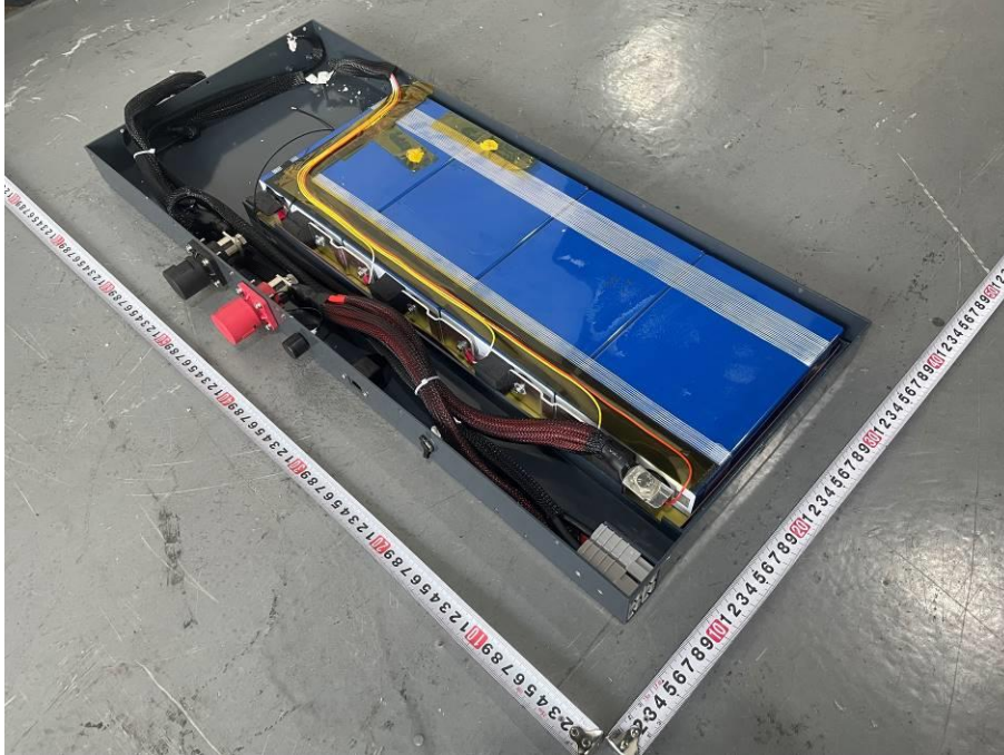
Figure 7 Internal view 3 of battery
